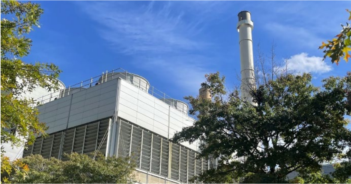
Figure 2: The lion's share of or electricity and space-conditioning needs is met by MIT's Central Utility Plant on Vassar Street (Photo: B Babakinejad)
