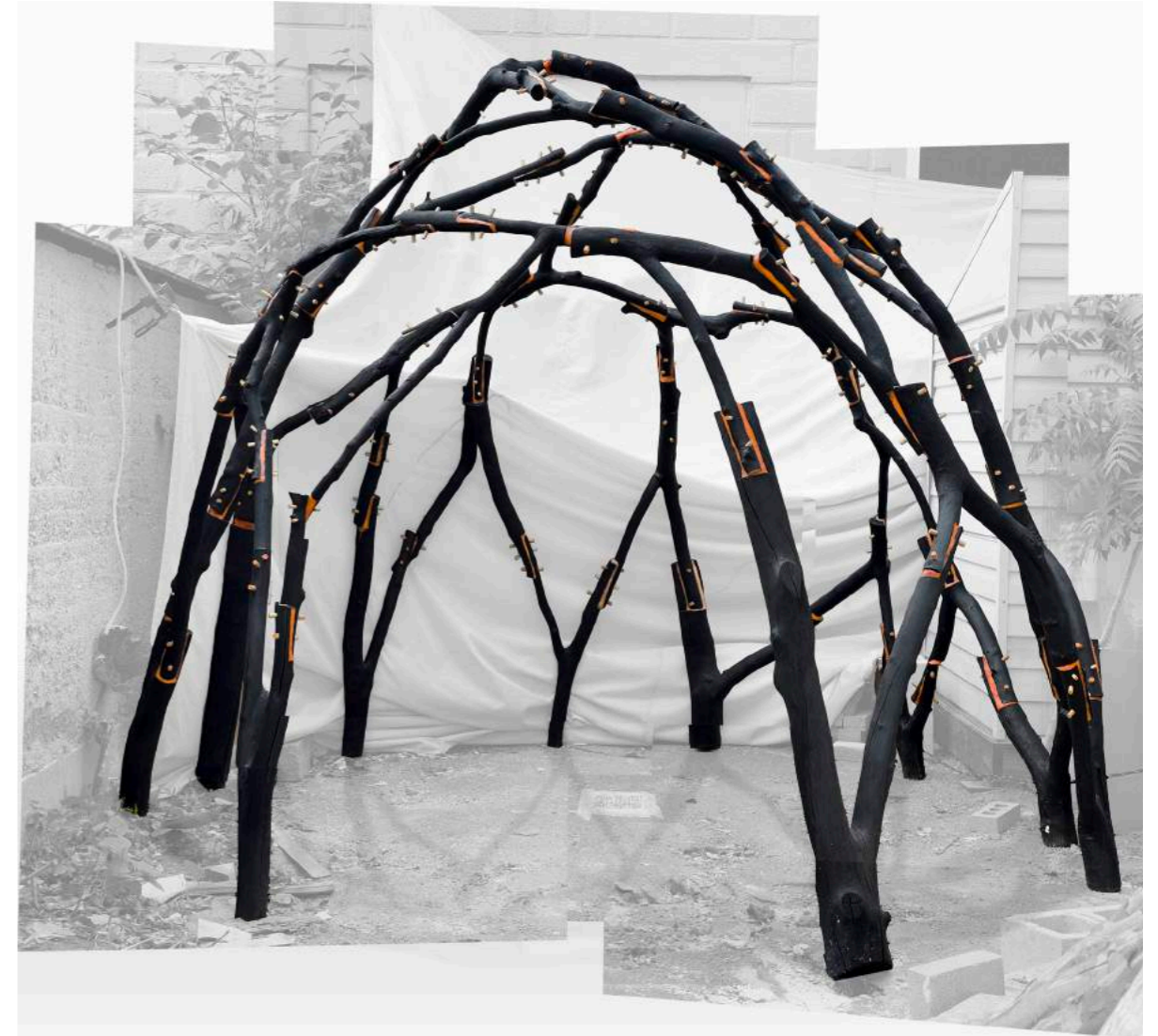
Wildwood Solar Kiln, currently under construction at MIT. The material library was sourced from trees recently cut down and pruned by the landscaping team to make space for a new campus building. The design was arrived at through the matching algorithm and optimization.
