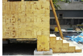
Entry stair added after manufacture and assembly of the cabin
